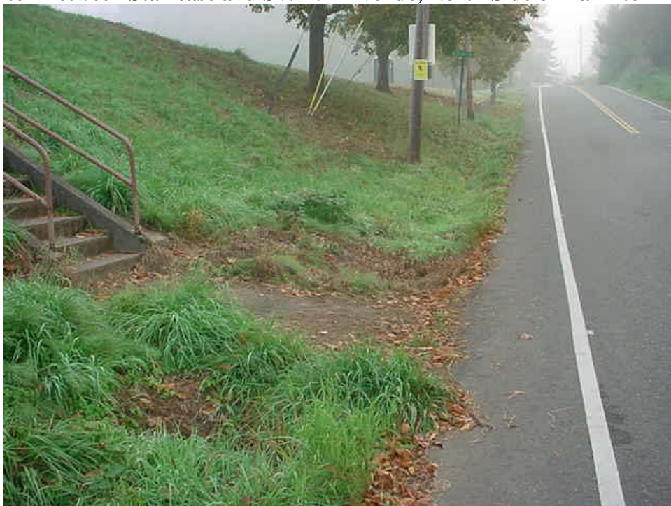
Figure 16. Ditch Between Staircase and SW 45 th Avenue, North Side of Hamilton
